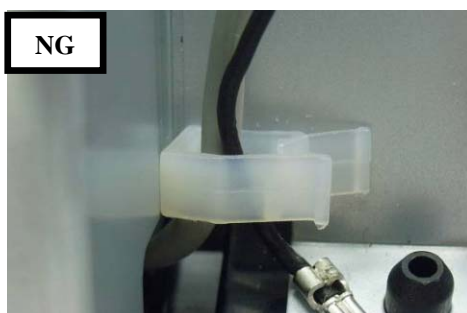
FG cable comes front of the shield wire.
